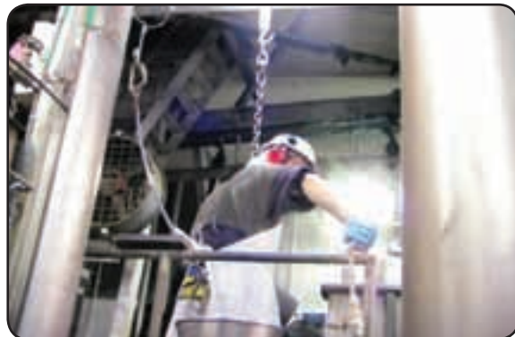
Example of waist belt harness with fall restraint lanyard attached to prevent the worker reaching the edge of the platform.
