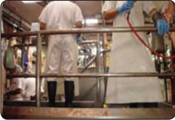
The use of handrails with a midrail and toe board as per AS 1657:1992 to prevent the fall of a person from this platform.
