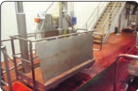
Rise and fall platforms fitted with appropriate railings and toe boards to prevent a fall.
